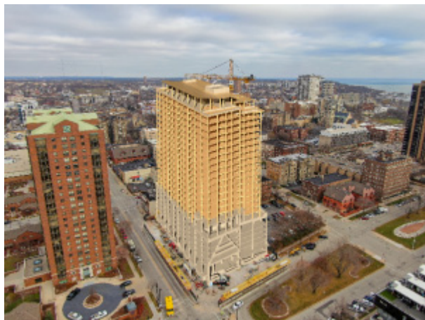
The 25-story Ascent Building under construction with mass timber products in Milwaukee, WI. Photo by Thornton Tomasetti and Korb + Associates
