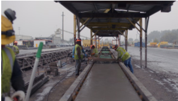
Precasting of cellulose-nanocrystal-infused concrete bridge planks. Photo by Michael Goergen, U.S. Endowment.
