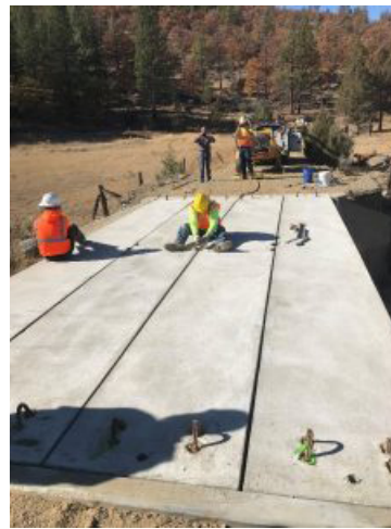
A bridge in California being constructed from cellulose-nanocrystal-infused concrete. Photo by Michael Goergen, U.S. Endowment.
